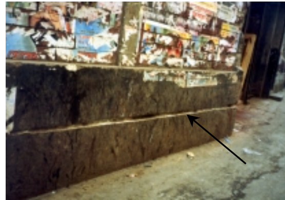
Fig.3 Damage of roadside wall, old part of Dhaka
